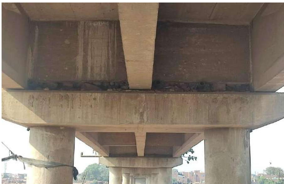
Figure 5-5 Deteriorated Bearing Plate
