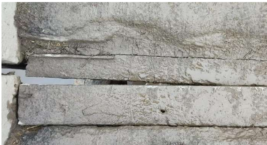
Figure 5-2 Defective Expansion Joint
