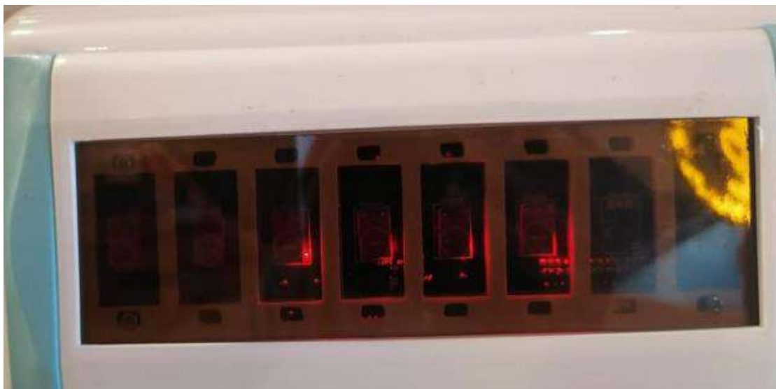
Figure 1: Wall Mounted Board
