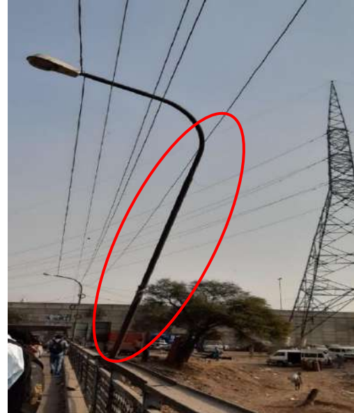
Figure 2.3 Tilted light poles
