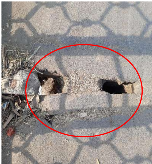
Figure 2.9 Damaged surface near joints
