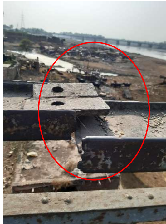
Figure 2.6 Missing Bolts at joints
