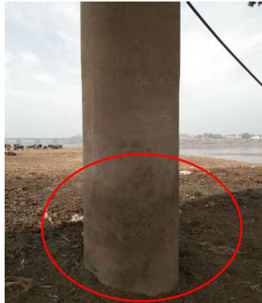
b) Unwanted material on pier stem
