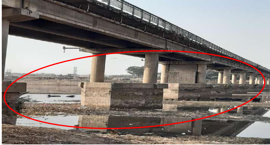
a) Pile caps having dampness
