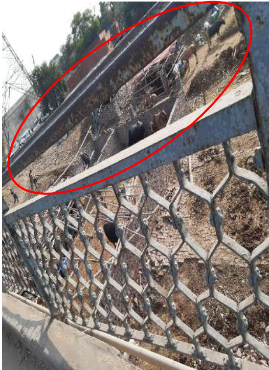
Figure 2.5 Corrosive surface of barrier
