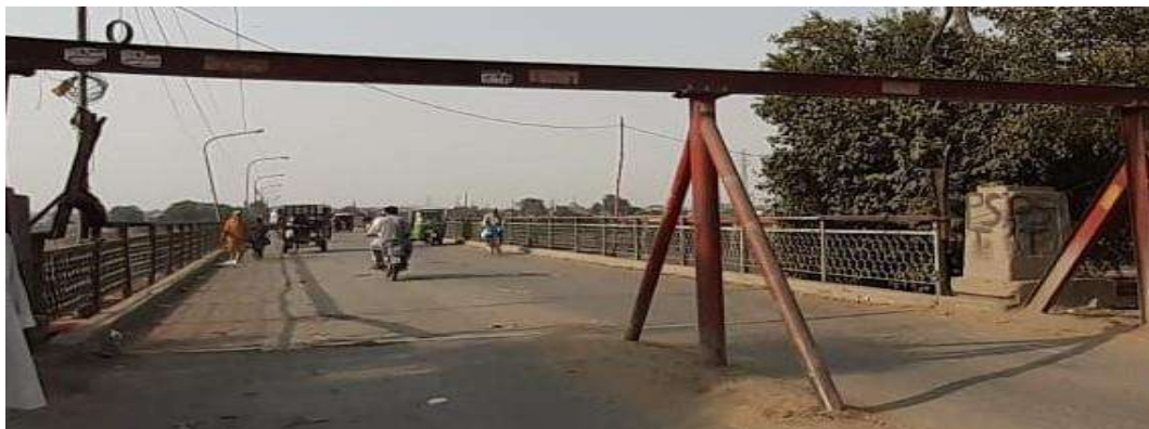
Figure 2.4 Barrier to indicate about load warning
