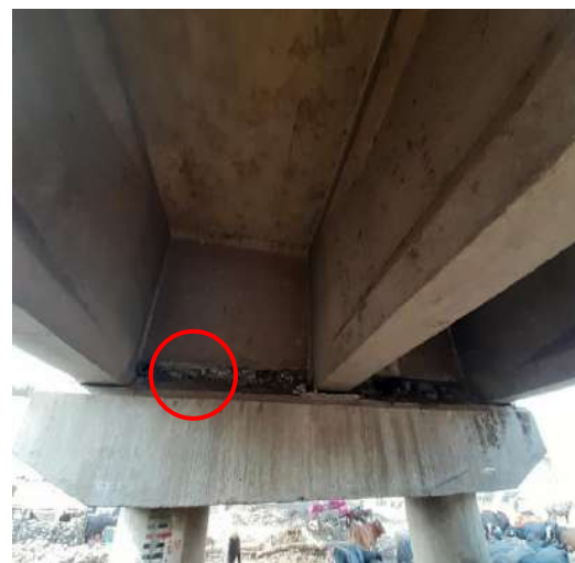
Figure 2.17 Unwanted and damaged pipes
