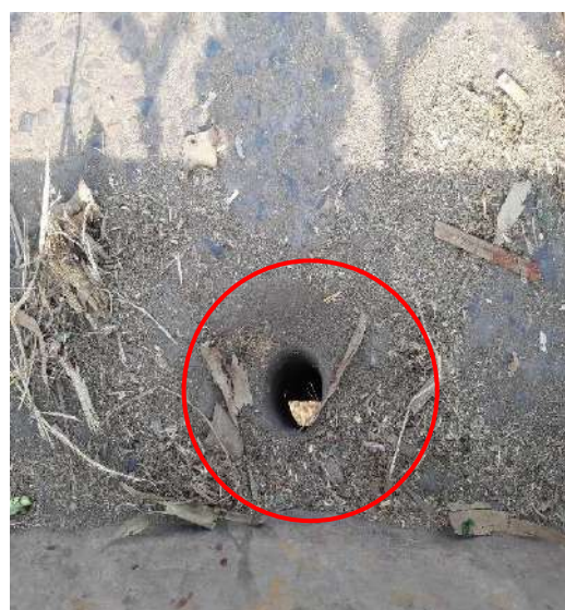
Figure 2.10 Holes in the wearing surface
