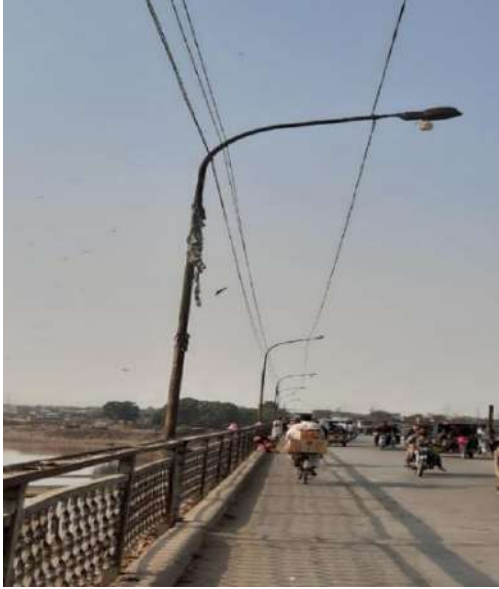
Figure 2.2 Straight light poles
