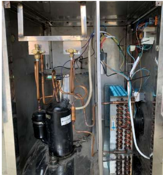
Figure 37: Internal view of heat pump
