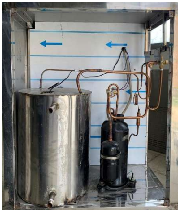
Figure 38: Internal view of heat pump
