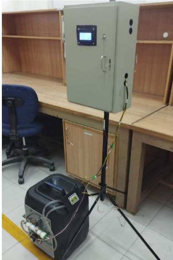
Figure 5.6 Complete Monitoring System in Running/Working Condition
