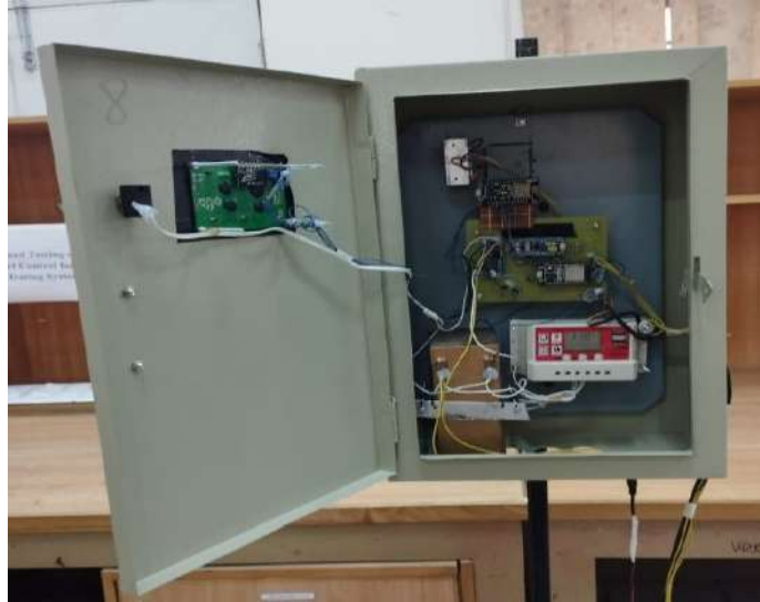
Figure 5.2 Inside View of Monitoring Box with Electronics
