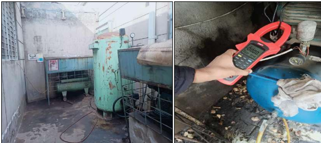
Figure 6.11: Compressor's rating measured by clamp meter.
