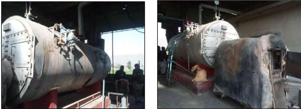
Figure 6.8: Installed boiler in the industry
