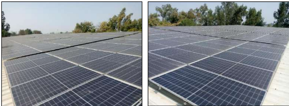
Figure 6.7 Installed solar system
