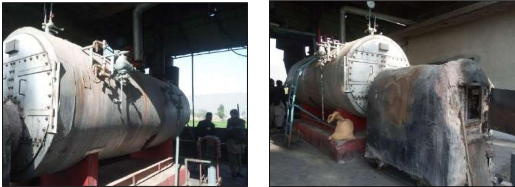
Figure 6.8: Installed boiler in the industry
