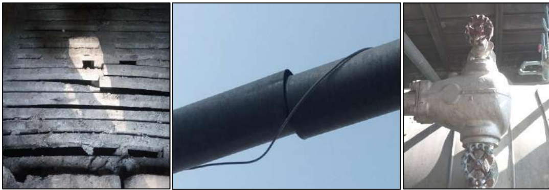
Figure 6.9: Broken components of Boiler
