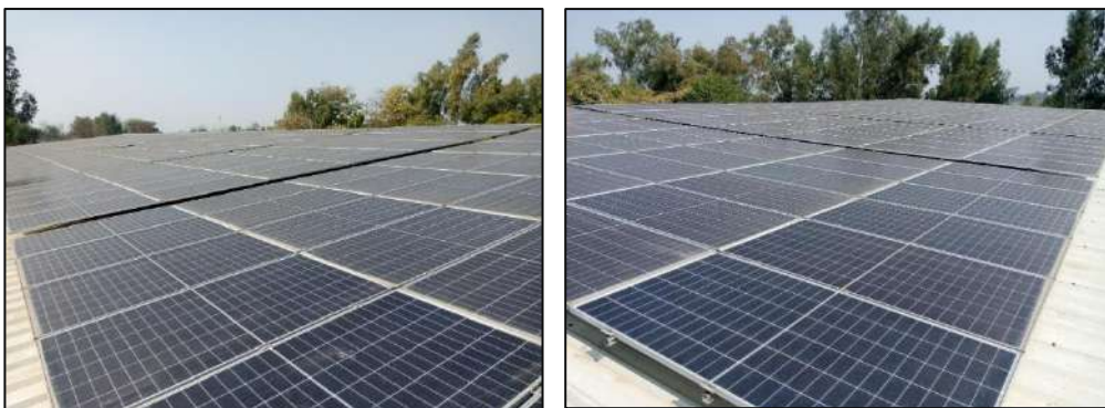
Figure 6.7 Installed solar system
