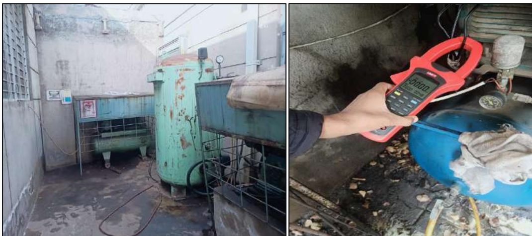
Figure 6.11: Compressor's rating measured by clamp meter.
