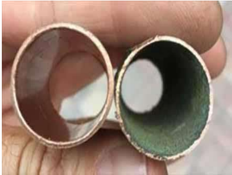
Figure 2 FOULING ON COPPER PIPE
