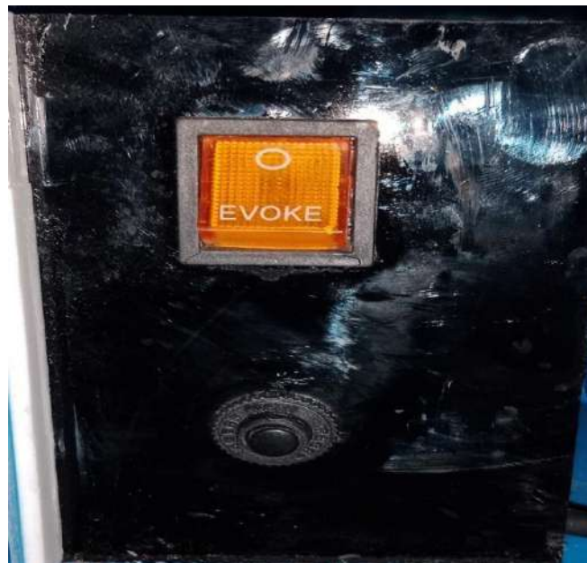
Figure 4-9: Emergency Shut down Breaker
