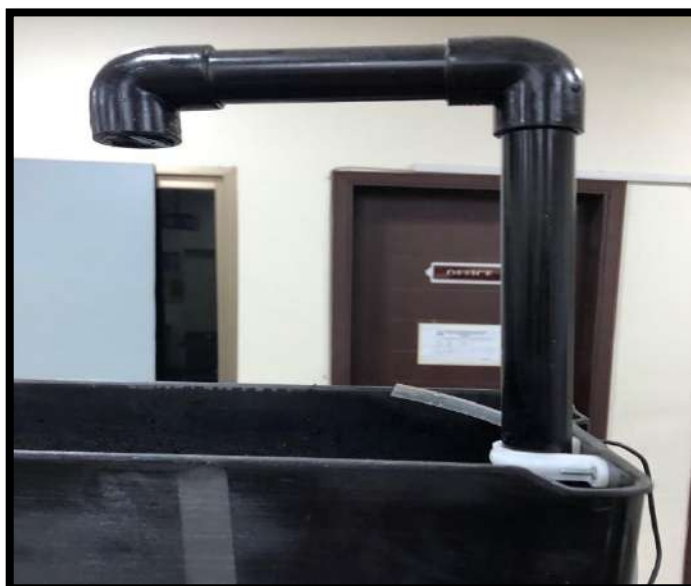
Figure 3.3(b): Ultrasonic Water Level Sensor Implementation
