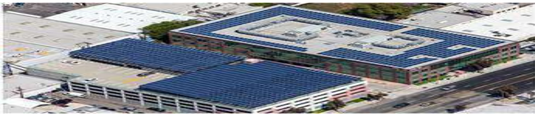
Figure 2.2(a) Commercial Roof-Top PV System 2
