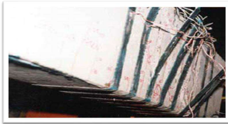
Figure 2.4 Debonding of FRP sheets
