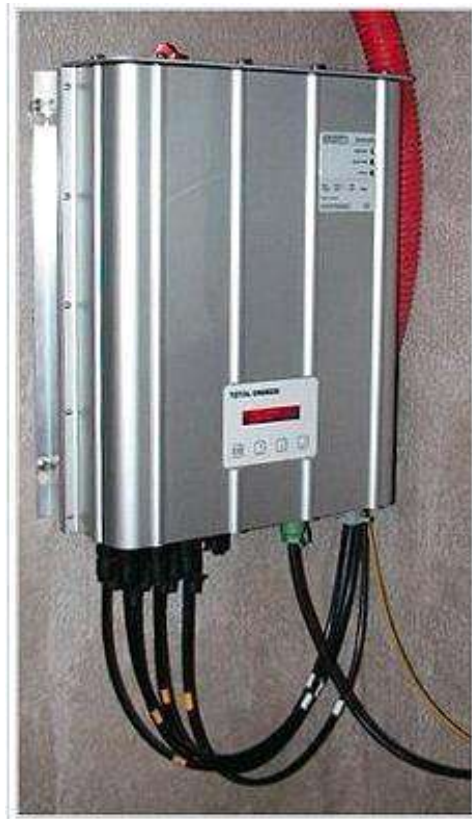
Figure 2.4 Inverter for grid tied solar panel.
