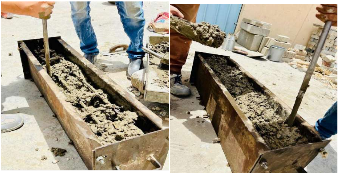
Figure 4.10: Roding of concrete
