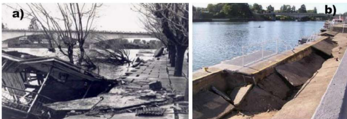
Figure 7: Liquefaction in Muelle Schuster at Valdivia city (Verdugo & González, 2015)
