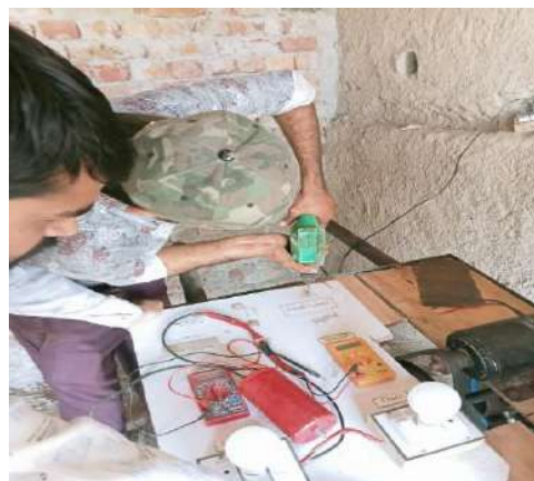
Figure 3-21: Fitting of Board with meters [18-10-22]
