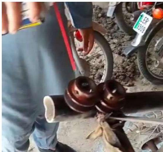
Fig 4.25: Spray on rusted pulleys [12-04-23]
