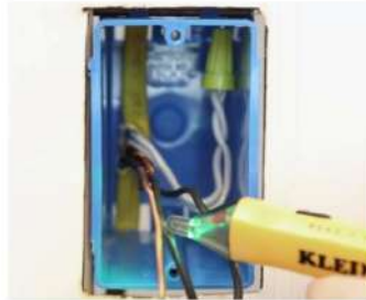
Figure 62: Detection of neutral wire using electric detector.
