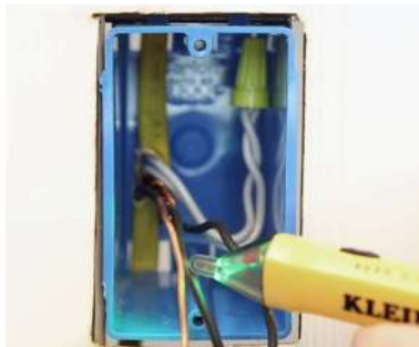
Figure 62: Detection of neutral wire using electric detector.
