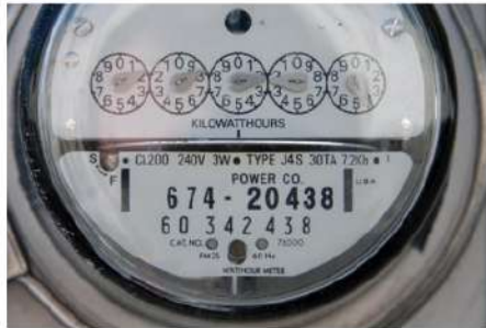
Figure 3: Analog Electric Meter
