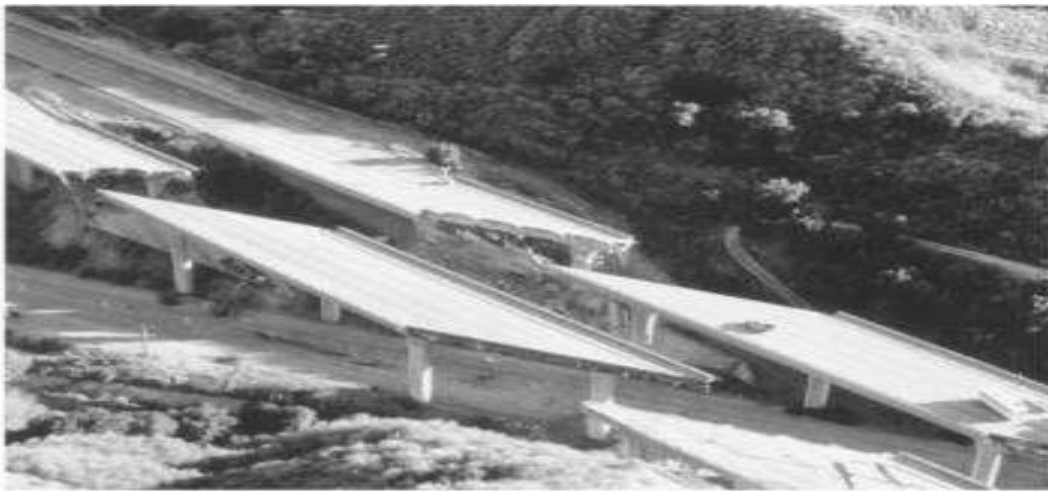
Figure 0-2: Gavin Canyon Undercrossing collapse in 1994 Northridge earthquake [10]
