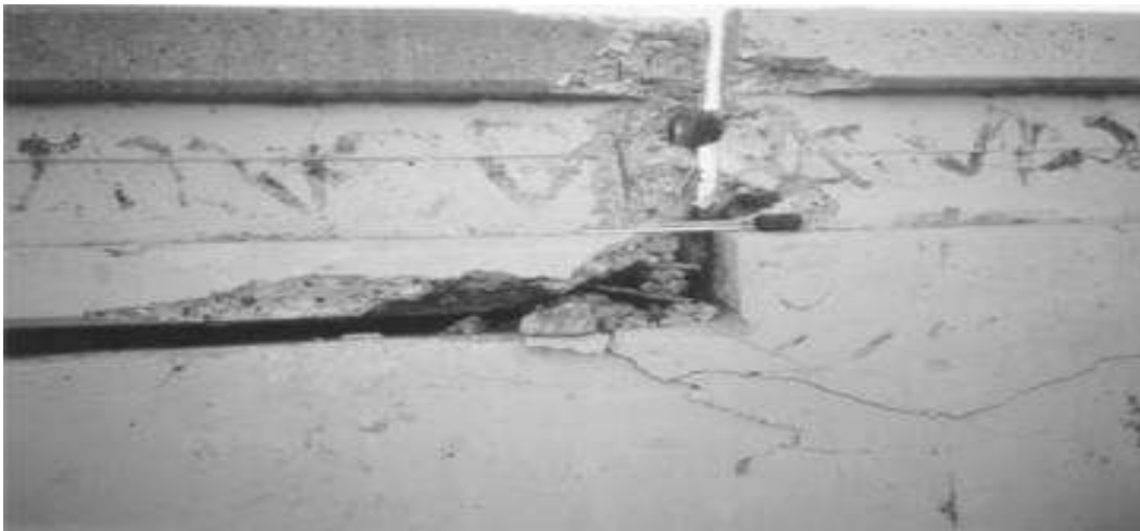
Figure 0-3: Santa Clara Bridge pounding damage to the abutment in 1994 Northridge earthquake [10]
