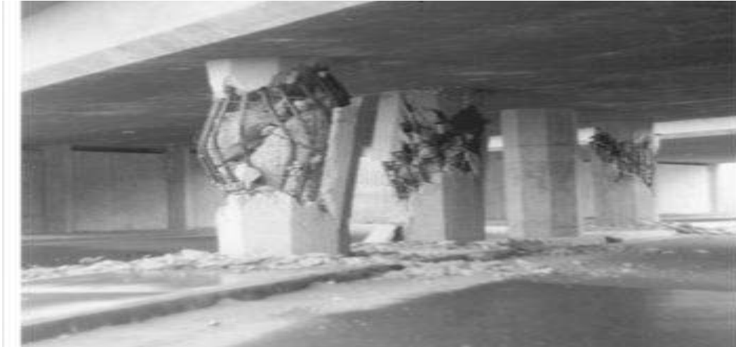
Figure 0-1: Columns Failure of the FBU [9]
