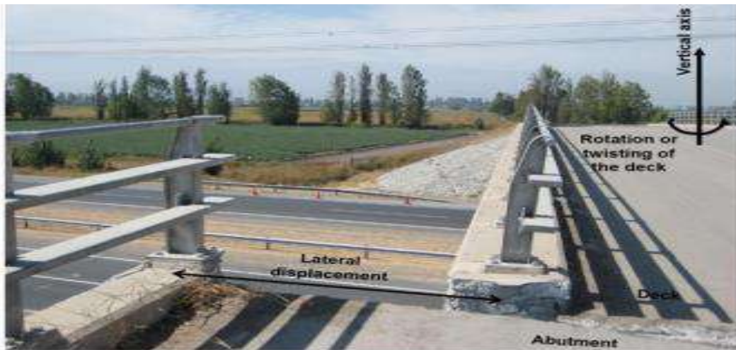
Figure 0-5: Damage to skew bridge after Chile Earthquake of Feb 27, 2010 [11]
