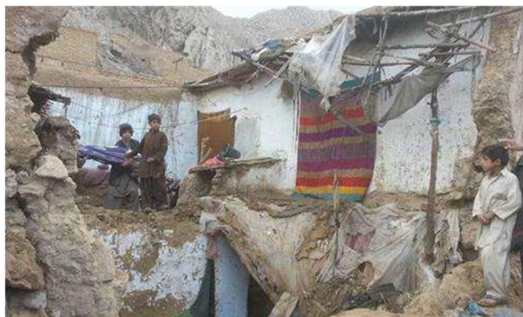
Figure 3.2 Failure of adobe structure after earth quake in Harnai in 2021
