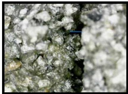
Figure 3.14a Crack at day 1
